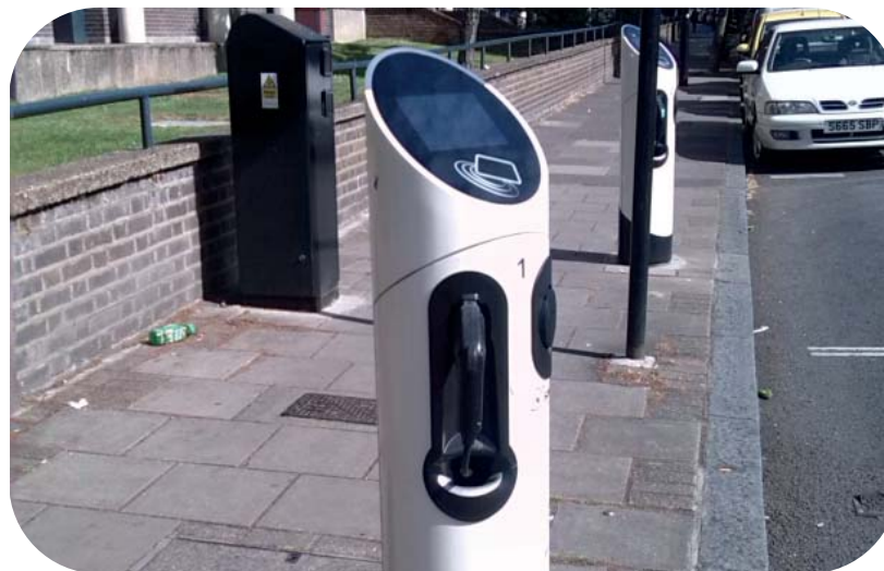
On-Street EV Charger
